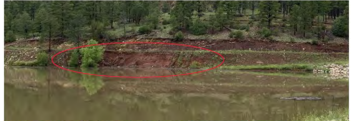
Westerly view of the diversion channel located along the west side of the Bradner Reservoir with eroded embankment slope as indicated.
