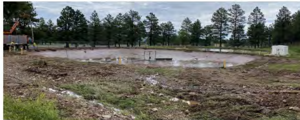
View of the inundated Water Treatment Plant Sludge Pond located to the north (downstream) of the Bradner Dam main embankment.
