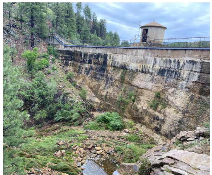
Figure 5 Peterson Dam After Overtopping
