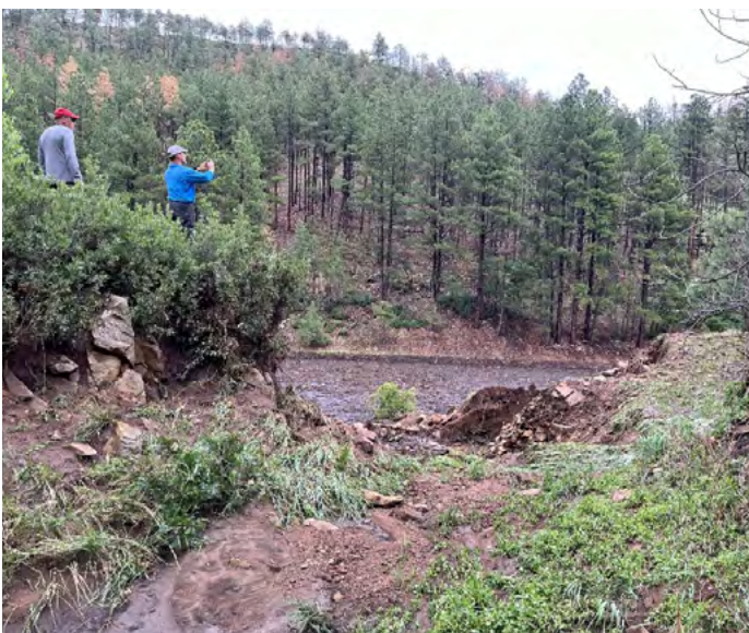
Figure 4 Breached Diversion Channel at Peterson Dam
