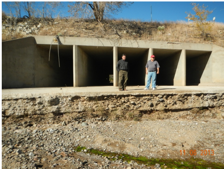
Figure 20 - Damage at the Village of Santa Clara, NM (Grant County), included 5 feet of downcutting immediately downstream of this box culvert.
