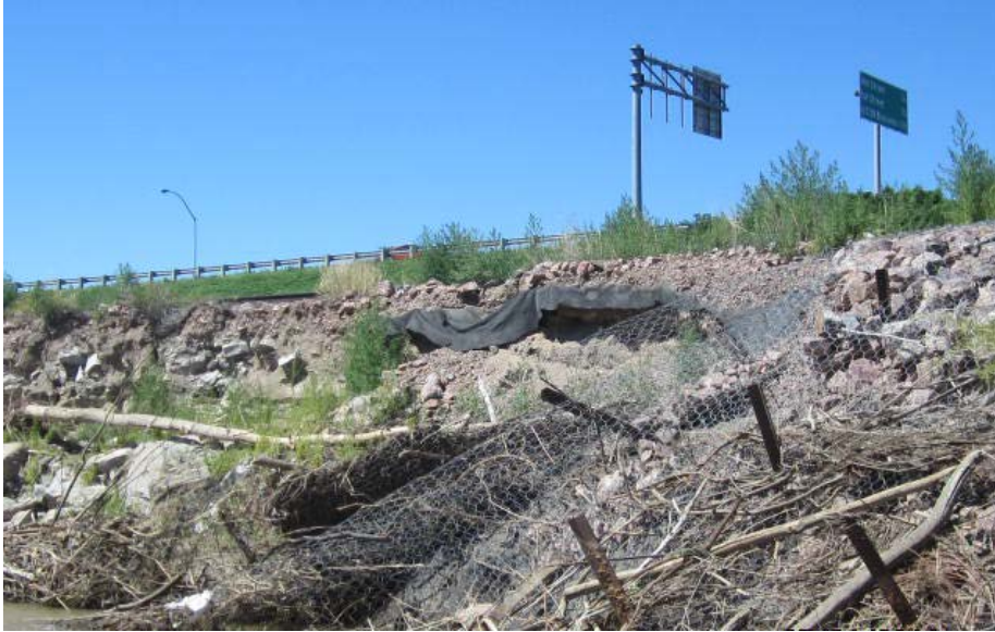
Figure 31 - Damage to railroad embankment along Fountain Creek in Colorado.
