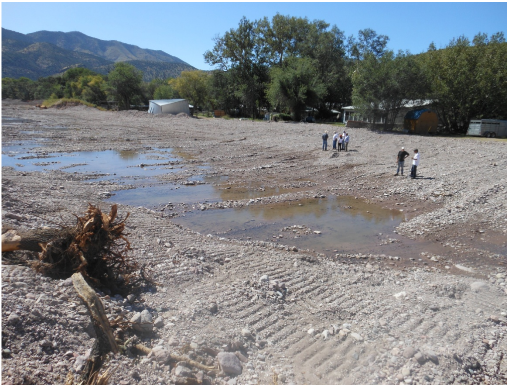
Figure 38 – Channel work along Whitewater Creek, near Glenwood, NM, following a September 2013 flood event.
