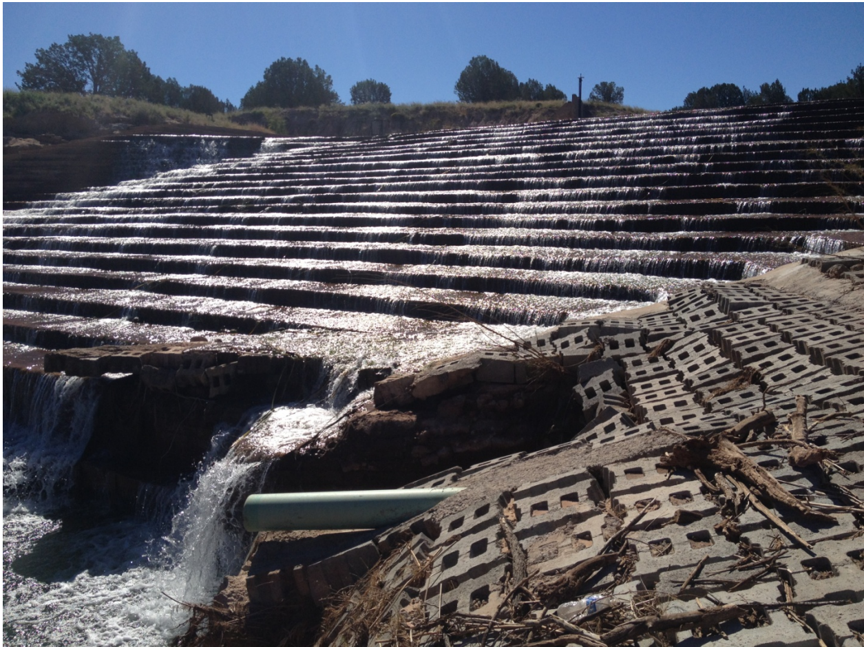
Figure 27 - Flood damage to the Giddings-Baca Diversion Dam, including erosion damage to the stilling basin and spillway toe.
