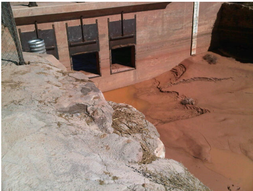
Figure 32 - Flood damage to a diversion structure in Many Farms, Navajo Nation (courtesy of Rose Whitehair).
