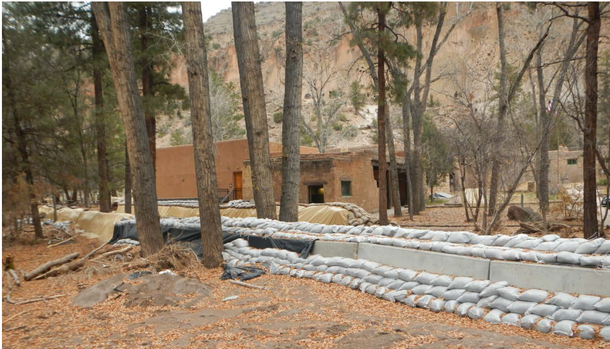
Figure 21 - Sandbags and Jersey barriers used to prevent flood damage to historic buildings at Bandelier National Monument.
